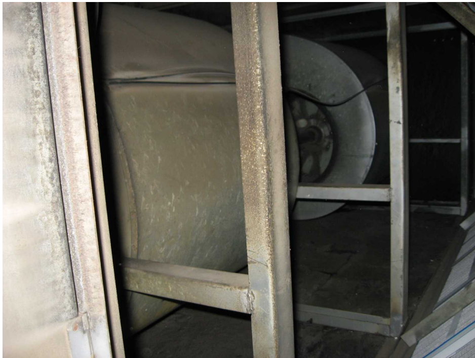
Figure 3-1: Existing Supply Fans in AH-2
